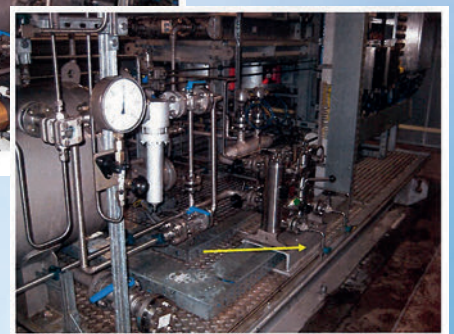
Figure 5: Location of manual drain point (Lube oil buffer/expansion vessel)
